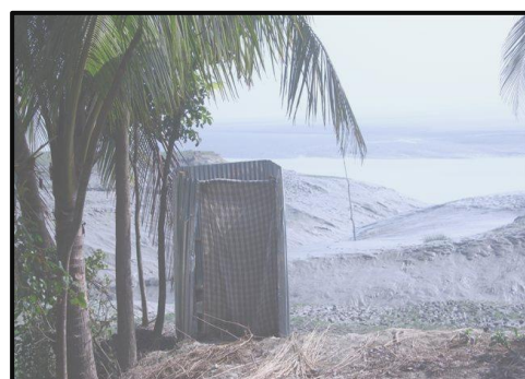
Photo 4.20 A weak structured ring slab toilet in Char Chandia
