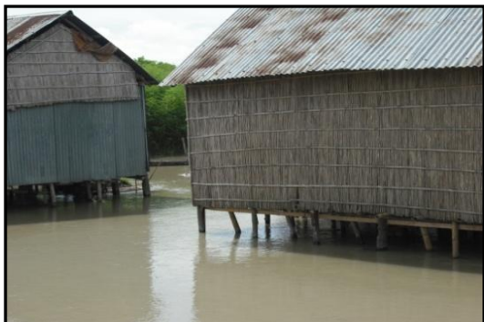
Photo 5.5 A flooded physical structure in Kunder Char
