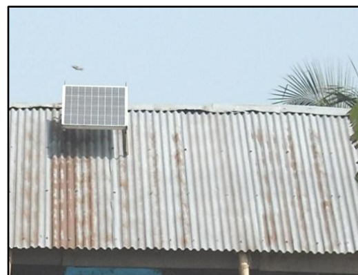
Photo 4.22 Roof top solar panel of a house of Kunder Char union
