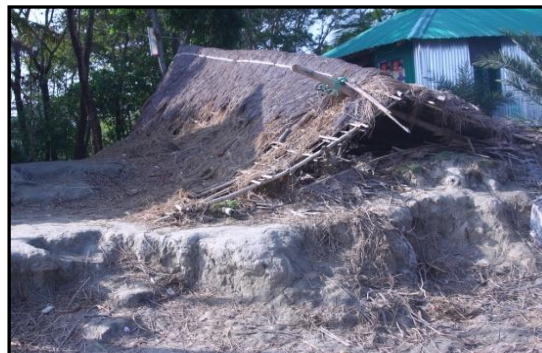
Photo 5.6 A house collapsed by cyclone Mohasen attack (05 May, 2013) in Char Chandia union
