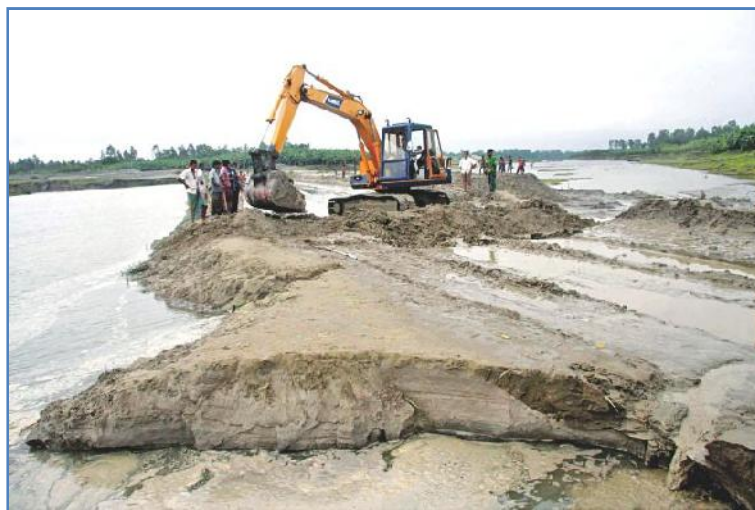
Figure 7.12 : Demolished road at Beltia village of Kalihati upazila in Tangail district.
