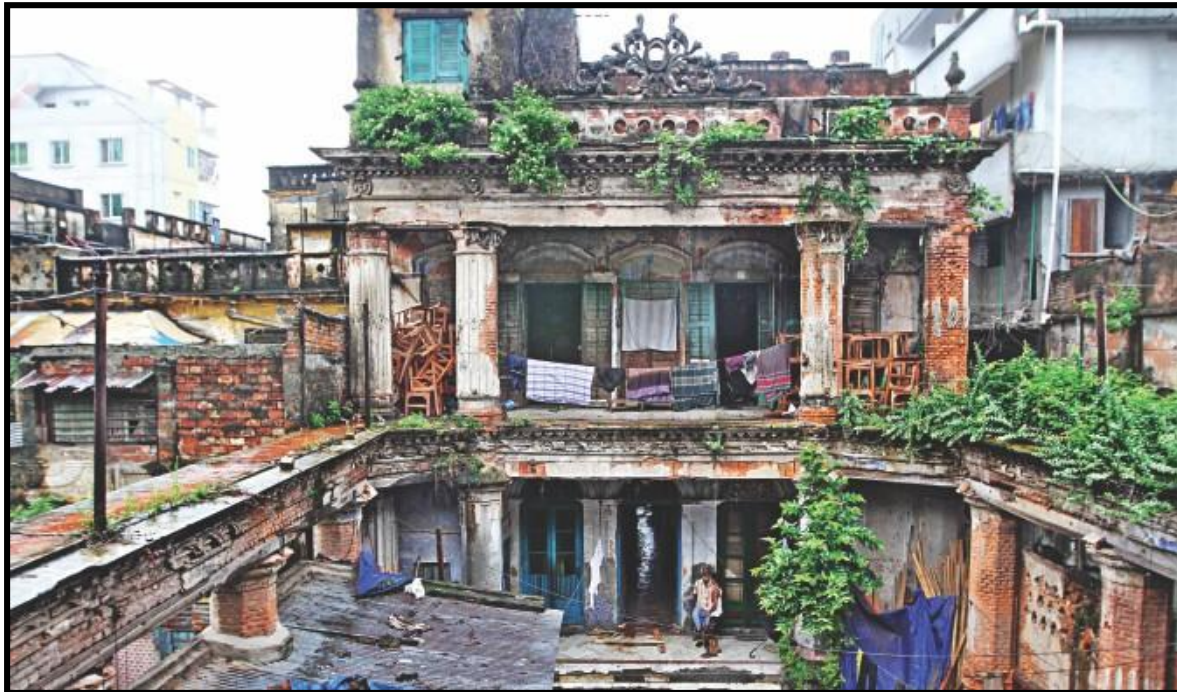
Plate: 22 A century old buildings in Old Dhaka, which speak of history, has archeological values but highly vulnerable to earthquake. Photo: Daily Star (March 08, 2015)
