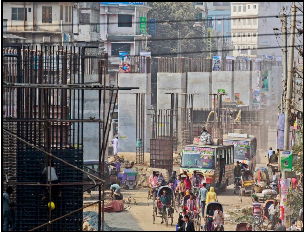
Plate: 7 Construction work of Moghbazar-Malibagh Flyover Project is going on in the capital.
