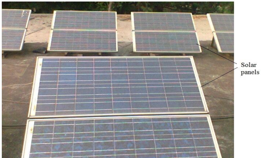
Fig-47: Solar panels on the roof top
