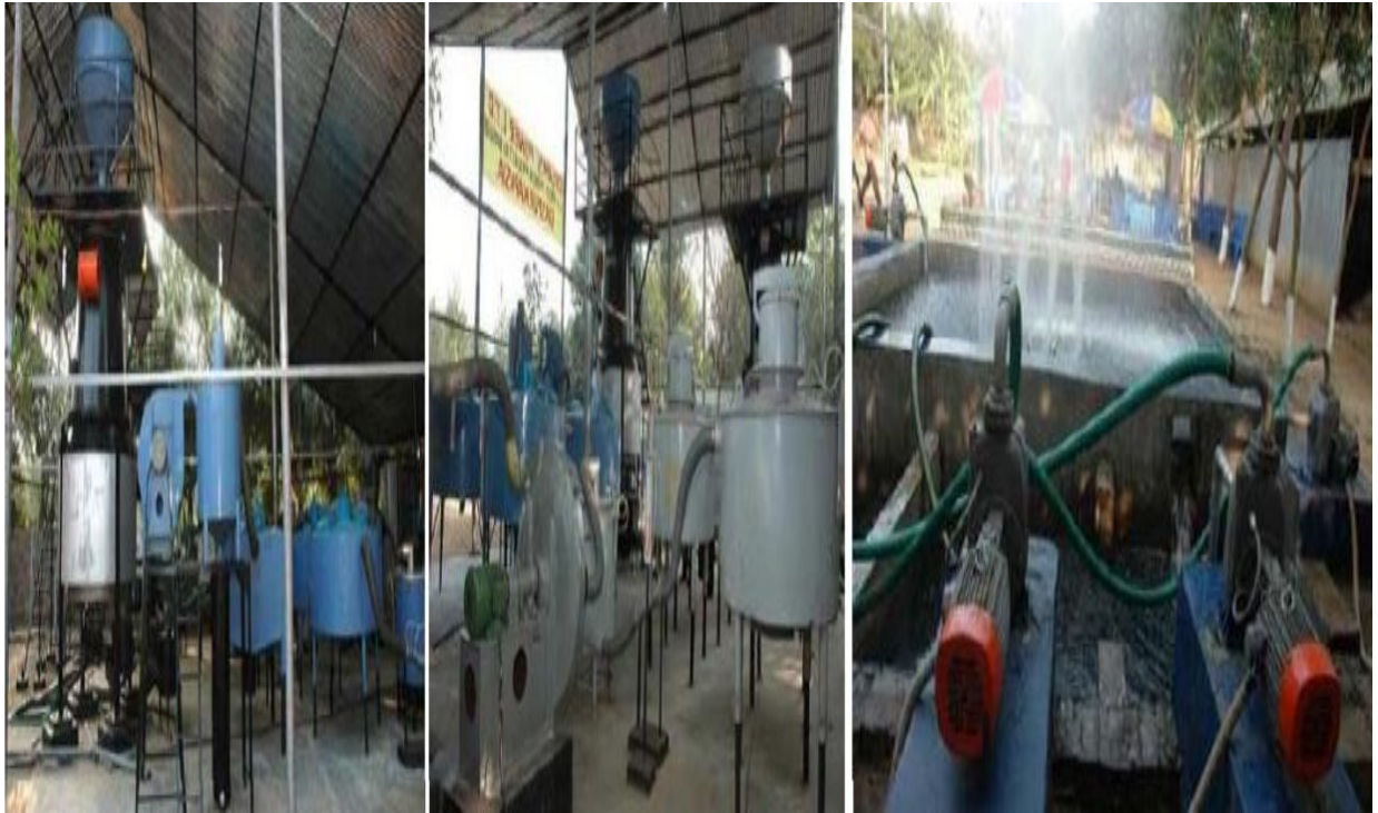
Figure 21: Rice husk fired 250 KW gasifier power plant at Kapasia, Bangladesh.
