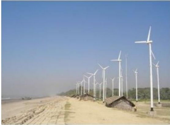
Fig(a): 900 kW Grid Connected Wind Power Plant at Matamuhuri Dam, Feni.
