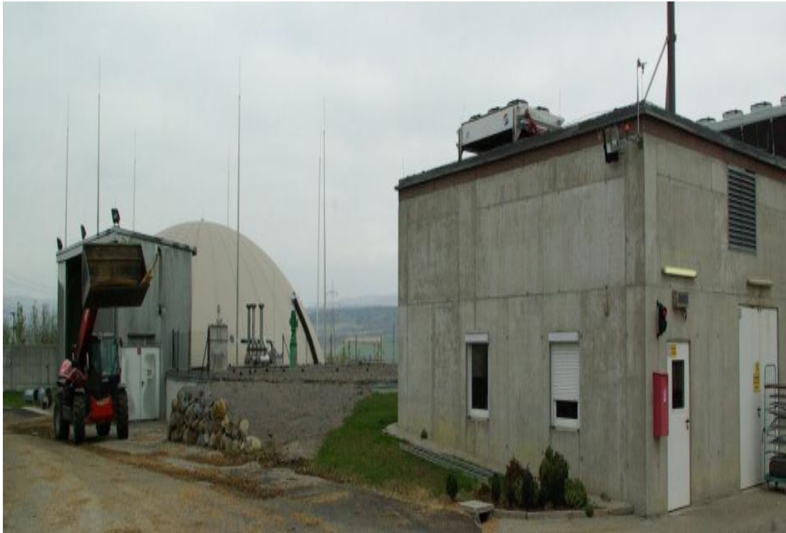
Figure 13: ElectraTherm Power+ Generator Installed at Biogas Plant in Austria
