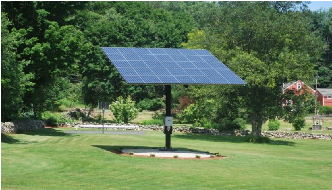
Figure 2.5 Tracker mounted photovoltaic [9]
