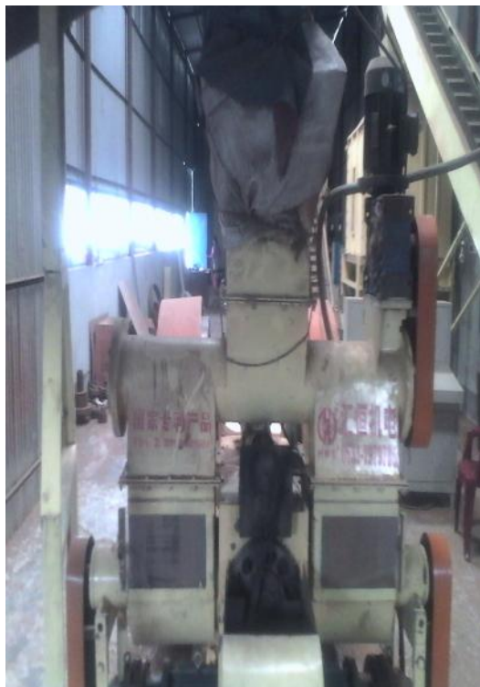
Figure 7.4: Pellet Processing Unit
