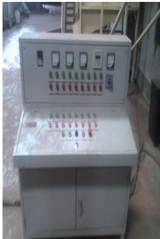
Figure 7.5: Pellet Processing Unit Control Panel
