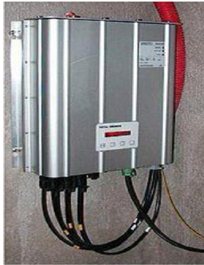
Figure2.6: Inverter for grid connected PV
