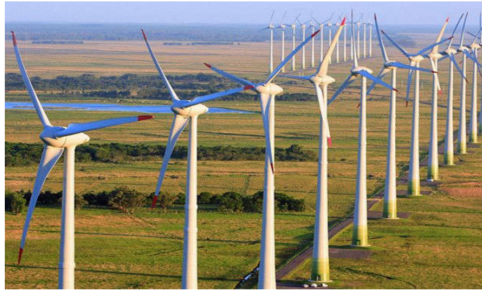
Figure 2-5 Wind Power Plant
