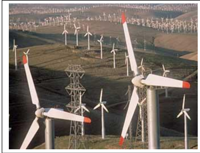
Figure 2.5: Wind Power Plant
