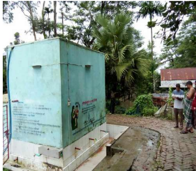
Fig 108: Drinking water storage from PSF in Patharghata
