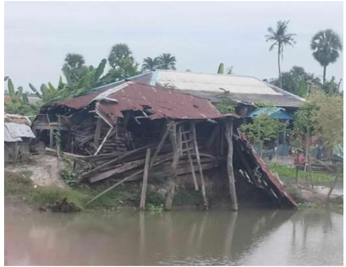
Fig 44: Destruction of Housing by cyclone at Protapnagar, Ashashuni, Satkhira
