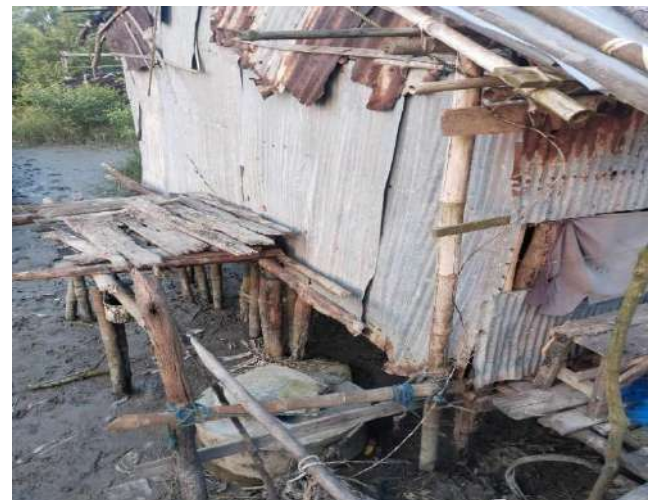
Fig76: Hanging latrine at Nalian village, Sutarkhali, Dacope
