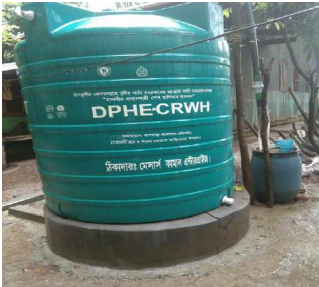
Fig 107: Drinking water storage in safety tank in Patharghata
