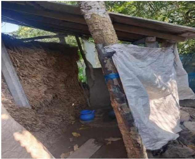
Fig 19: Sanitation system at Tengrakhali, Shyamnagar, Satkhira
