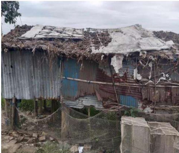
Fig 45: Weak housing condition at Kurikahunai, Ashashuni
