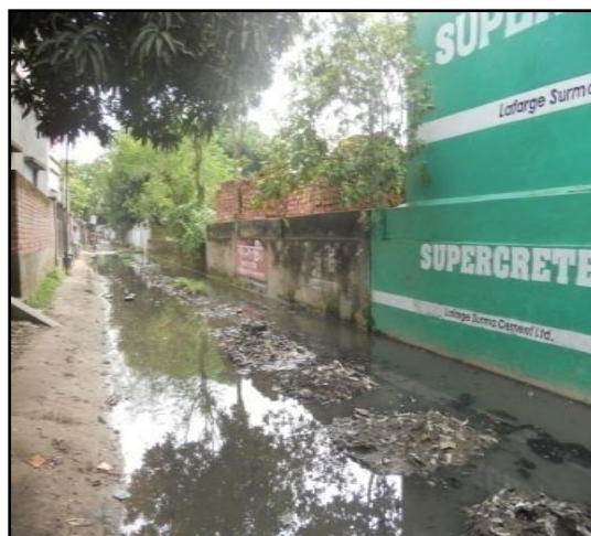
Picture: 5.6 Water Logging Situation due to Drainage Blockage
