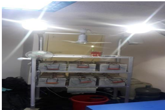
Figure 2.18: Front side experimental setup of a 1 KW PKL /AL power plant
