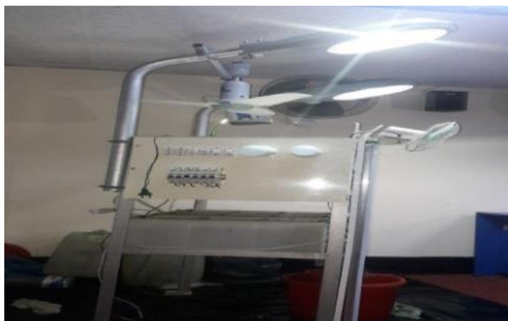
Figure 2.19: Left side 1 KW PKL power plant
