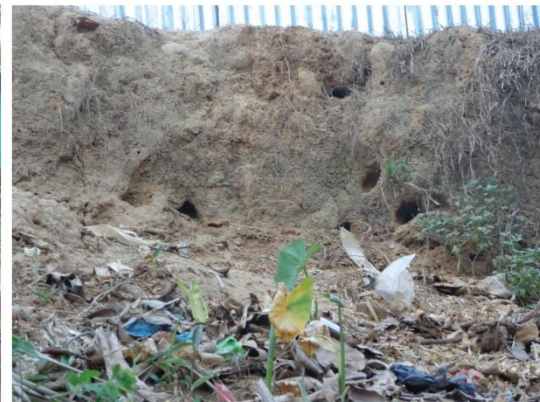
Photograph: 30 Soil erosion adjacent to housing in Rangapani
