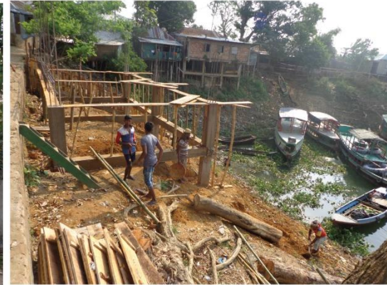
Photograph: 36 The house under construction adjacent to the lake on the side of the road in the old slum.
