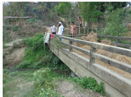
Photograph: 24 Unplanned bridge cause by flood on Manikchari
