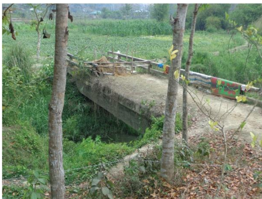
Photograph: 23 Unplanned bridge on Manikchari canal Which is causes of flood
