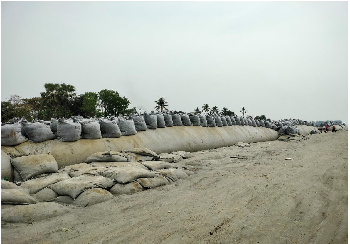
Figure 7.2 Sand-filled geo-bags to protect the fragile sea beach, March 2021 (Source: Picture taken by the researcher)
