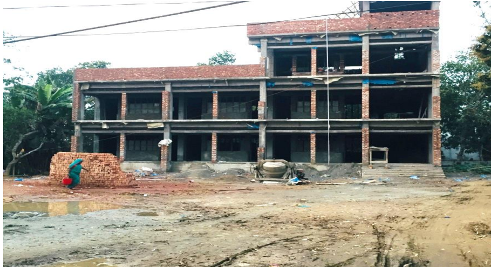
New building under construction of Dangora primary school by the government support
