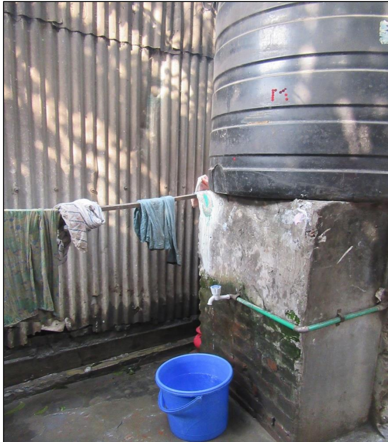
Photograph 2a: Electric tube well/borehole with tap (Private installation)
