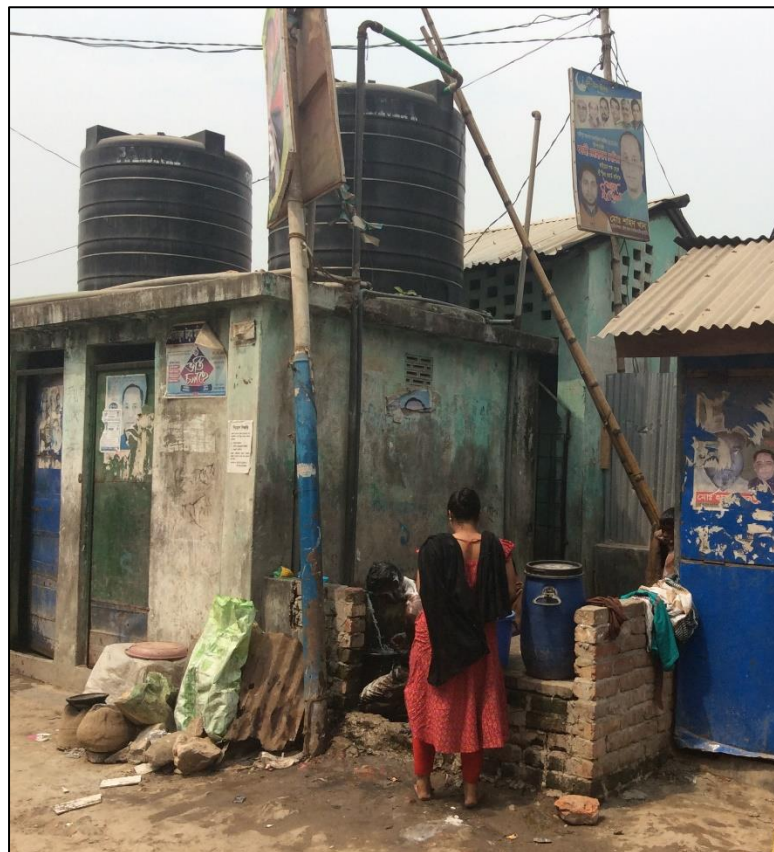
Photograph 2b: Electric tube well/borehole with tap (Group or community installation)
