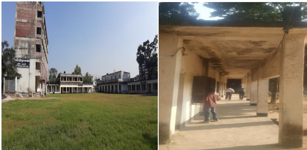
Fig. 4.13 School Buildings Vulnerable to Building Collapse
