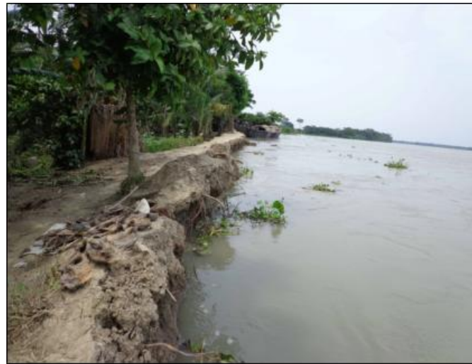
Picture 6: Faulty management of embankment and river erosion if favorable to salinity intrusion
