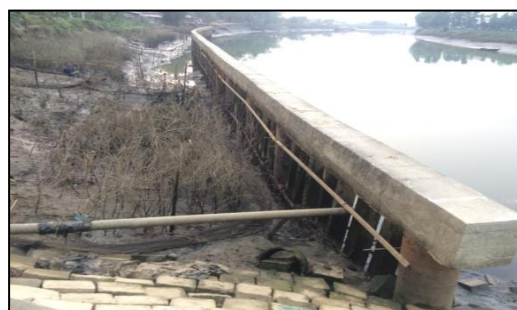
Illustration 8.14: Shoreline erosion protected with spurs at upstream of Bakkhali River Rubber dam, Cox's Bazar, 2017
