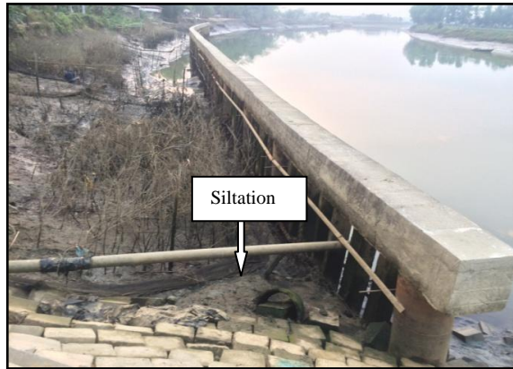
Illustration 8.17: Siltation inside the Spurs along the downstream of Bakkhali Rubber Dam, Badar Mokam, 2018
