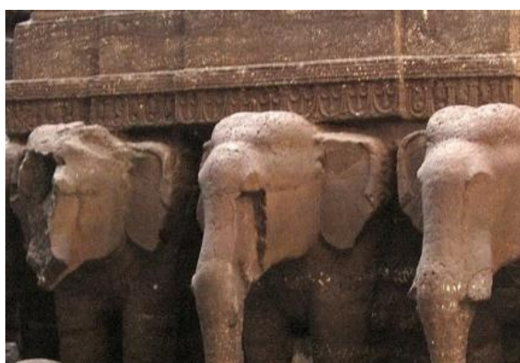
Figure no.- B10. Festoon and marginal can be observed in the elephant platform of Kailasa Temple
