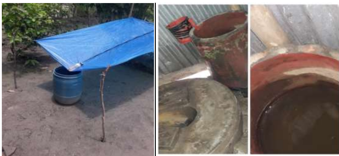
Picture-3: Saline water used in the washroom in Sundar Mahal Picture-4: Rainwater harvesting system in Sundar Mahal
