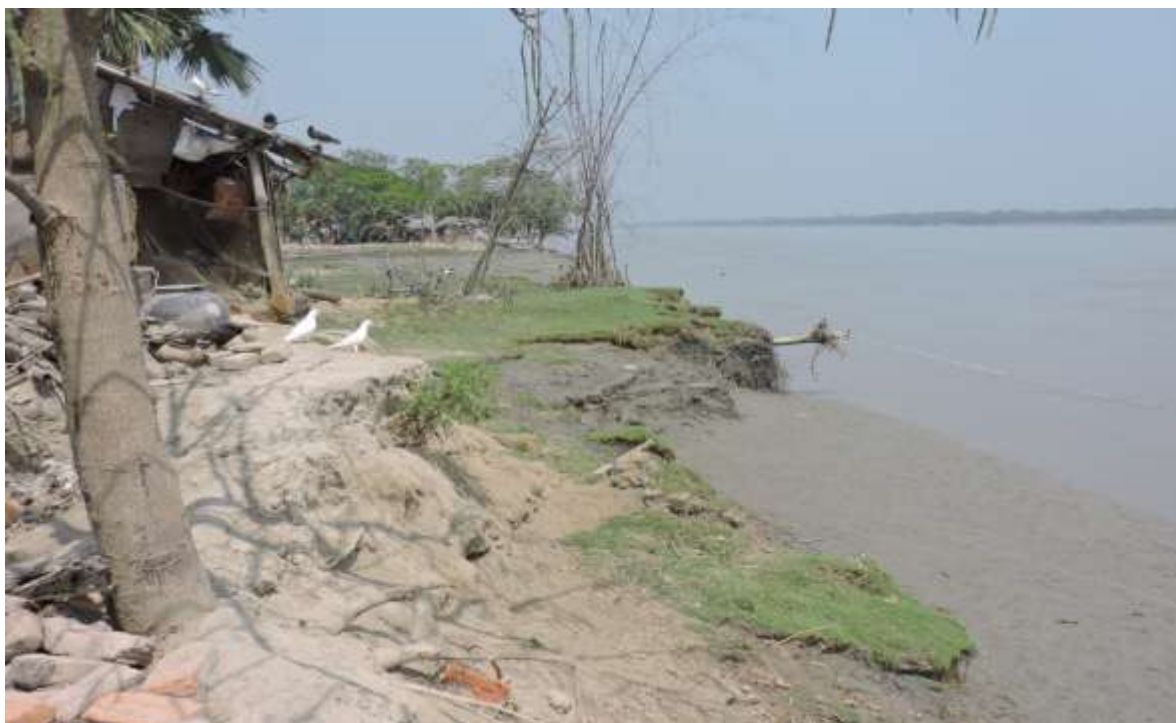
Picture-11: The Impacts of river erosion in polder 29
