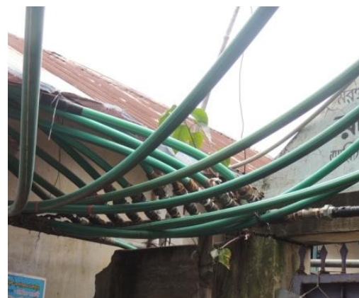
(iv) Aboveground network pipe
