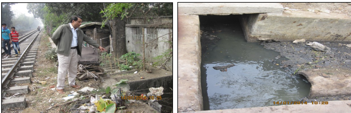
Figure 4.1: Connection of polluted lake water under the drainage of Banani railway area
