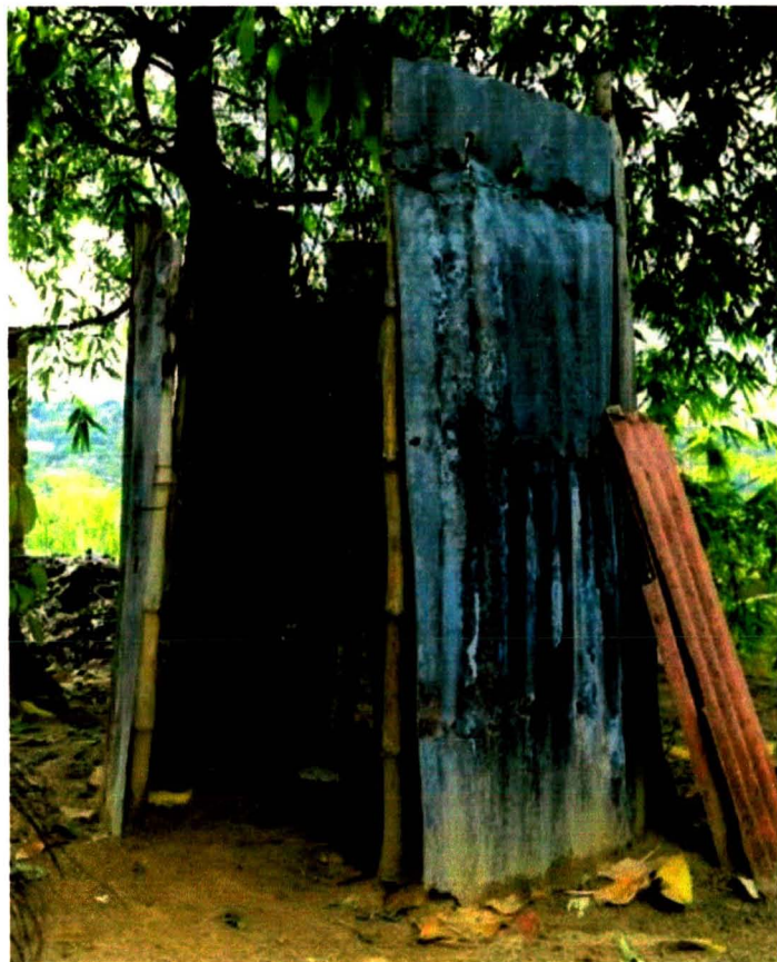
Fig 65 . Insanitary toilet (Page no.- 8 )
