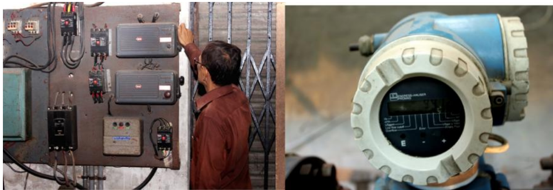
Fig21.Machines used to supply water to head tank Fig 22. Two pumps were used
