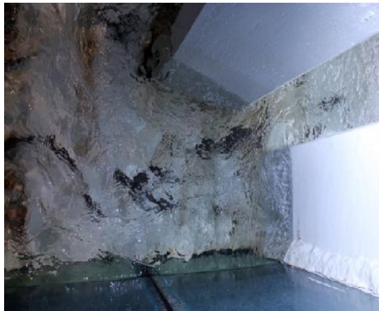
Fig 107. Water flow inside the fish pass
