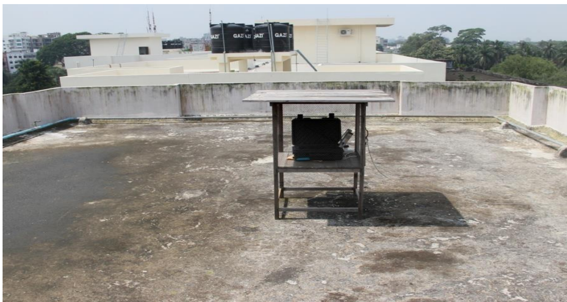
Figure 3.3: Photographs of the toxic gas monitoring instrument installed at the roof-top (20 meter above ground level) of the “House Tutor Quarter”, Amar Ekushey Hall, Dhaka University, Dhaka, Bangladesh. The same instrument was used in all the locations for trace gases measurement.
