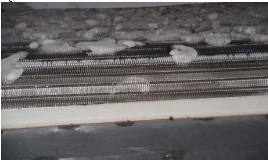
Fig 2.25. Chill water machine
