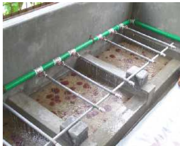
3F Continuous water flow
