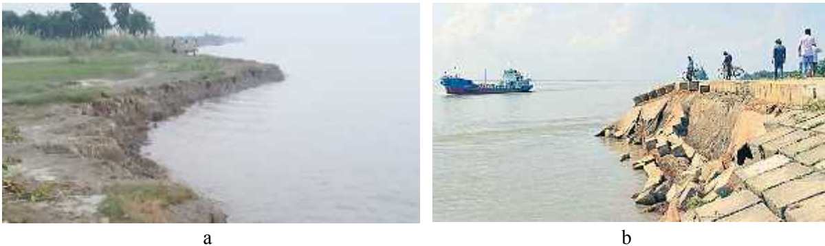
Figure 28: Riverbank erosion in the study area: a) Riverbank erosion in Dhulsura and b) riverbank erosion in Andharmanik
